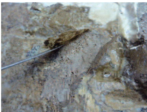
Adhesive on the surface
